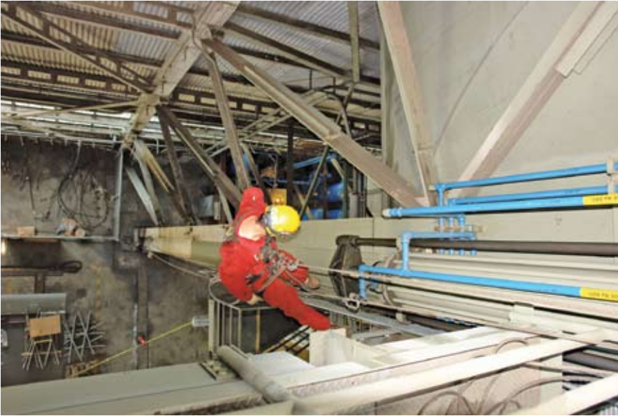
Besides inspecting vane sets in the NFAC wind tunnel, the RAT crews also performed work on other hard-to-reach systems, such as the actuating components of the 40- x-80-ft test section overhead doors.
