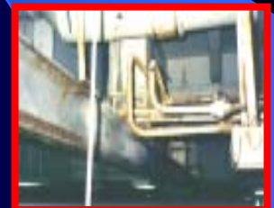
Well-Deck Overhead with MIL 24441 System
