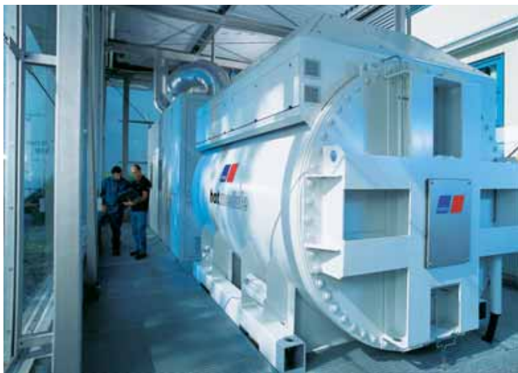
The HotModule fuel-cell power plant is the result of 10 years of development work and, according to MTU CFC, should be ready for series production in 2006. It generates electricity as well as process steam from manufacturing facilities.
