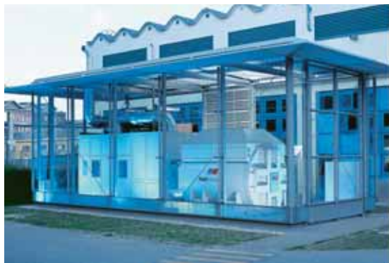
The first MTU CFC bi-fuel fuel cell went into service at Vattenfall Europe AG in Berlin last year. It is fueled with natural gas or methanol or any mixture of the two. The methanol used is derived from waste generated locally.
