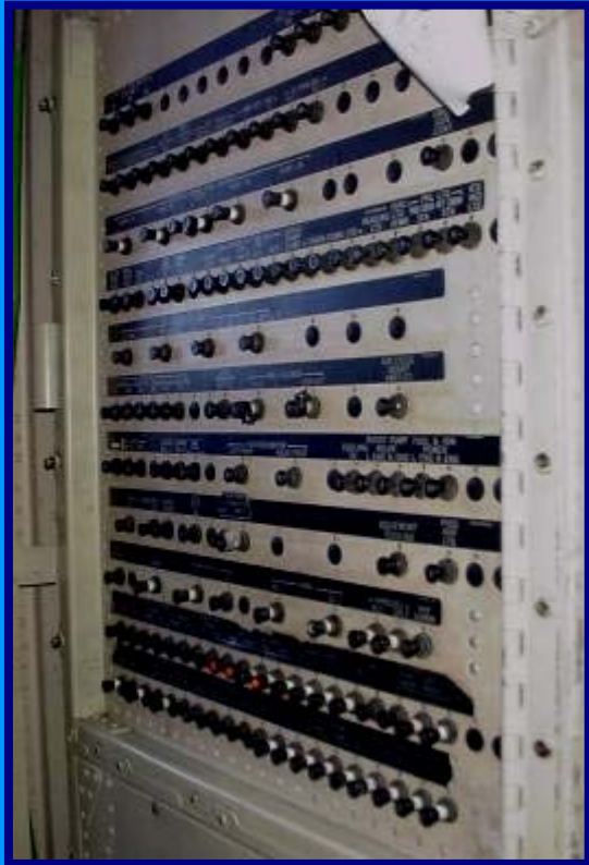
EA-6B Circuit Breaker Panel Testing
